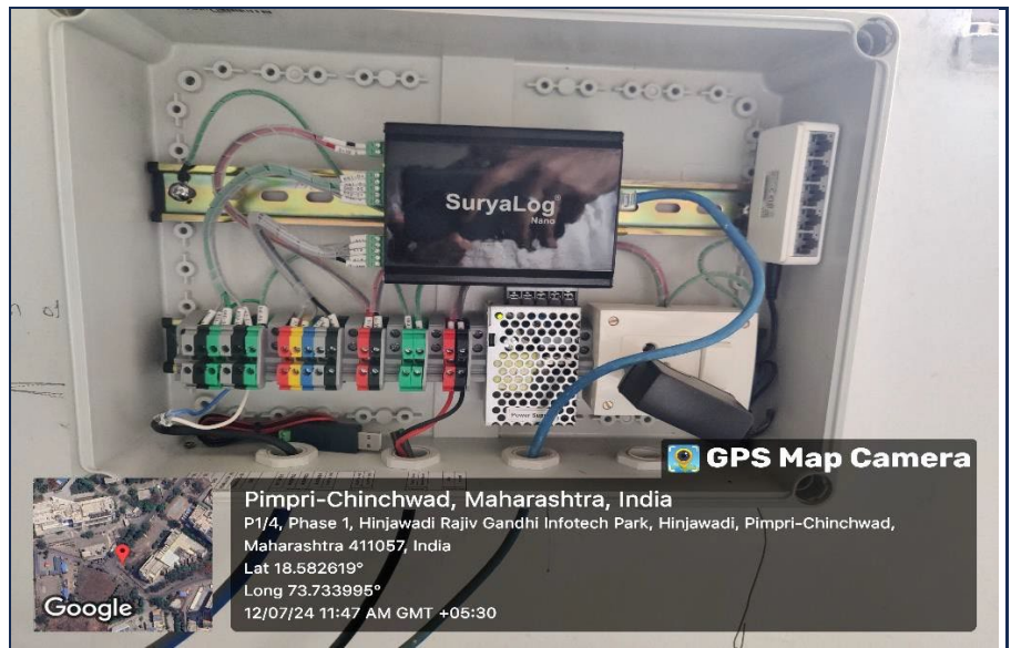
Fig 4. The Energy Monitoring System in the panel room
