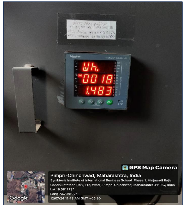
Fig 2. Grid Energy Meter near MSEB panel for input for EMS
