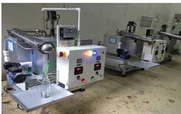
Plastic (PP & PE) and waste oil processing reactors to generate hydrocarbons
